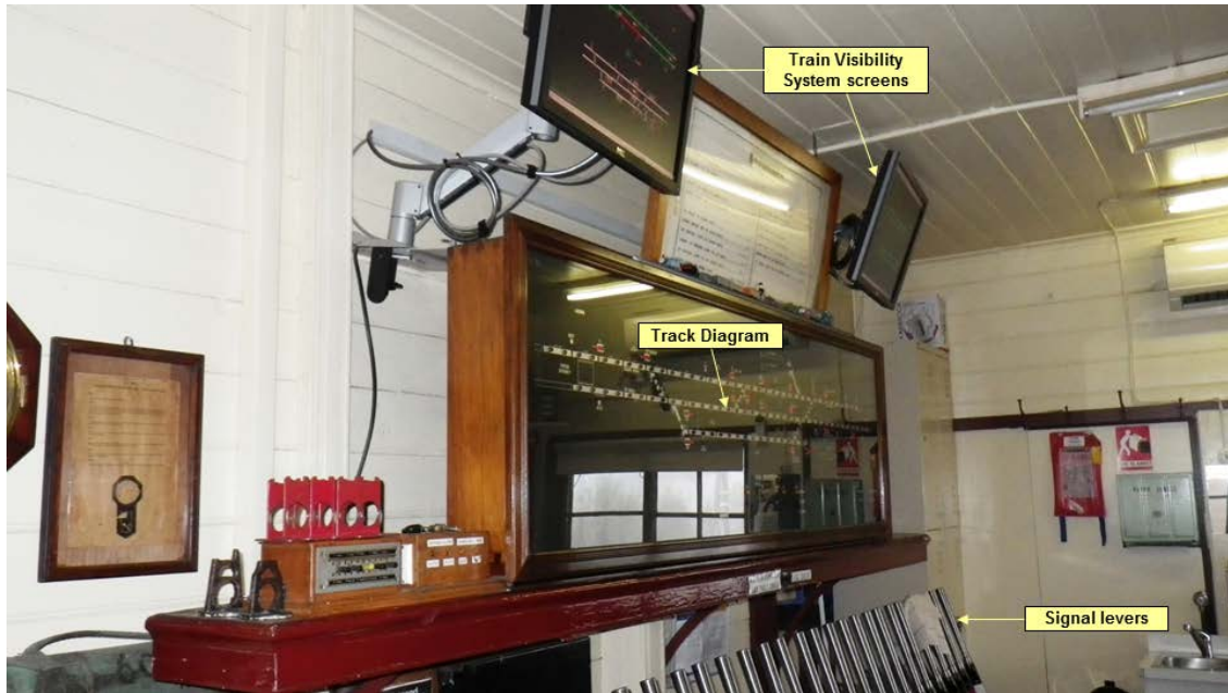
Figure 5: Katoomba signal box
