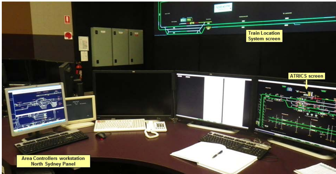
Figure 7: Homebush signal complex – North Sydney control panel
