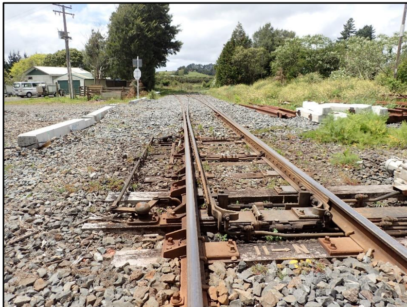
1.1 points, Paerata, showing the route for the setback movement to the Branch Main (left)
