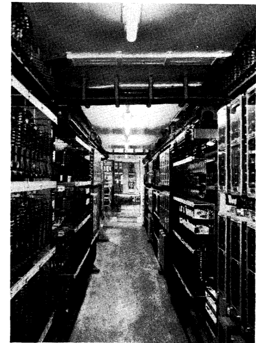
Fig. 10 Interior of relay room under operating room, Geneva panel installation
