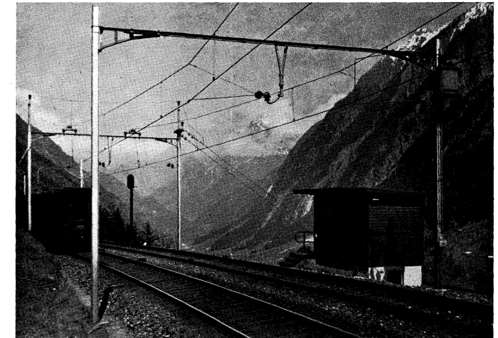
Fig. 14. Automatic intermediate signal location at Eggwald on the Gotthard line, showing axle counting impulse magnets on track
