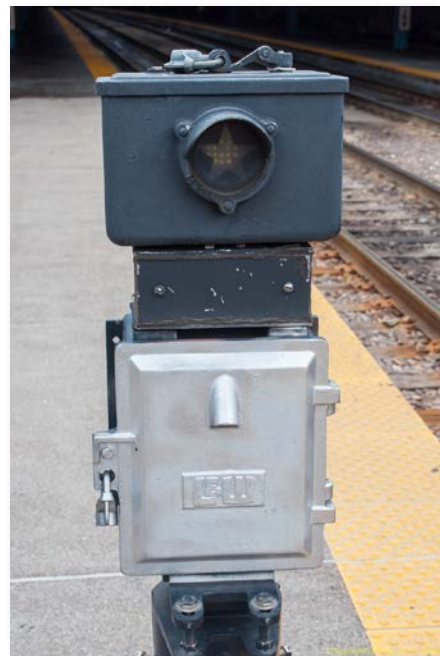
Rear view of signal 131 showing the back light referred to in the special instructions. This light illuminates only when the corresponding signal displays an indication more favorable than Stop .
