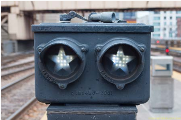
A close-up view of the lamp unit containing the two star indications on the front face of signal 131. These stars are permanently illuminated, and simply identify the corresponding signal as the first signal governing movements from each of the train shed tracks and therefore subject to the special instructions. Observe that the stars, like the main aspect of these signals, are illuminated using an array of light-emitting diodes (LEDs) that produce lunar white light.
