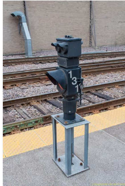
Side view of signal 131. The stenciled numbers are used to help identify each individual signal; after all, there are a total of 67 dwarf signals in the Lake Street interlocking plant!
