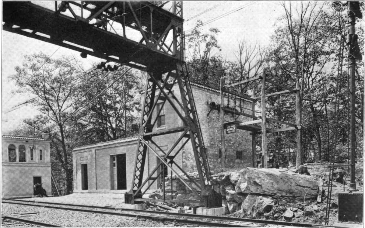
Fig. 13. The Signal Sub-Station, Showing the Entrance of the 11,000-Volt Mains.
