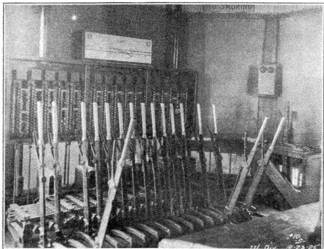
La Rose interlocking machine with covers of special circuit controller cabinet, in rear, removed
