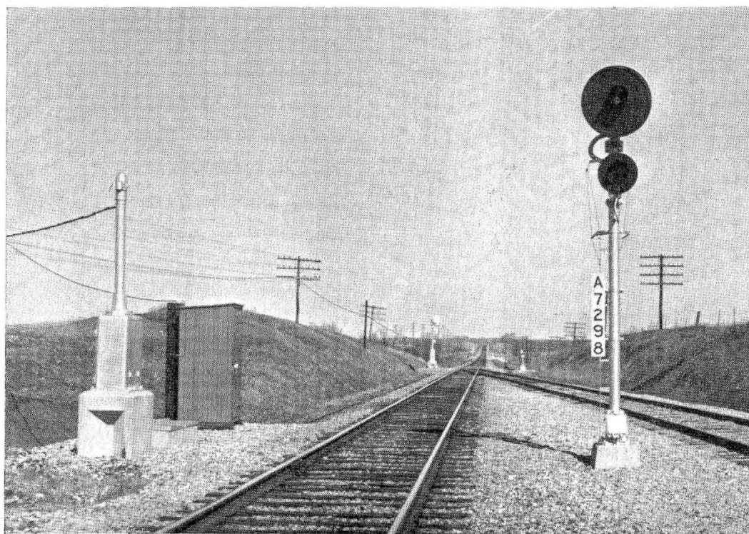
The new automatic block signals are located so that no changes would be required when changing to C.T.C.
